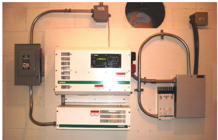
The indoor monitoring system for the solar panels.
